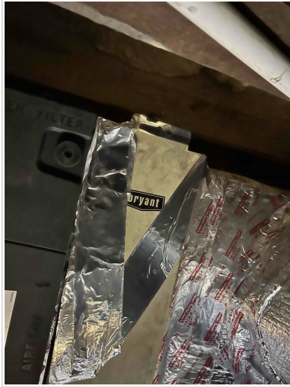
Door to filter cabinet
